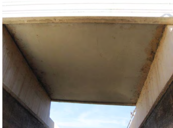
Photo 3-81. No cracks or spalls were observed on the underside of the pedestrian bridge.
