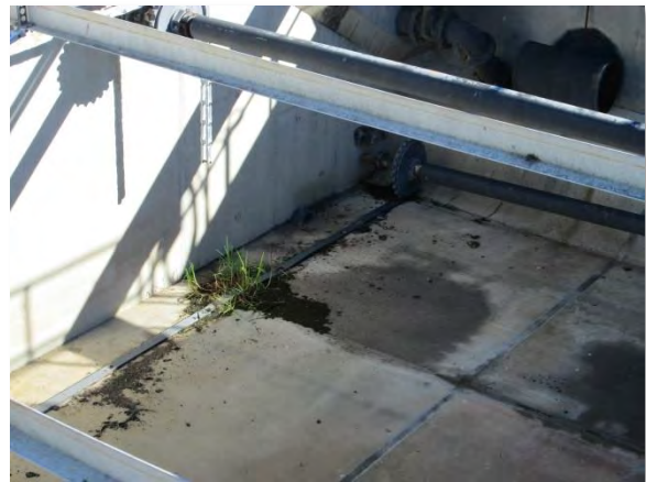
Photo C-33. Weeds growing from expansion joints.
