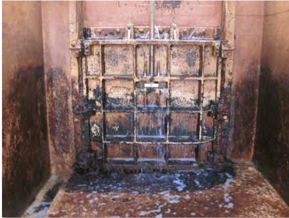
Photo 3-86. Outlet sluice gate at northeast corner of CCC was leaking.
