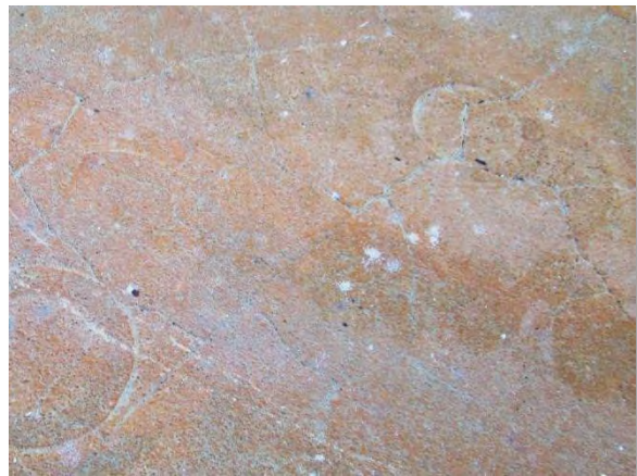
Photo A-24. Typical cracks in PC 1 floor.
