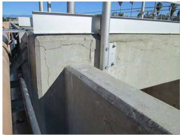
Photo C-2. Cracking on edge of walkway.
