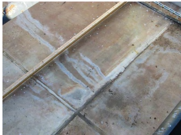
Photo C-29. Gaps in expansion joint sealant with possible seepage.
