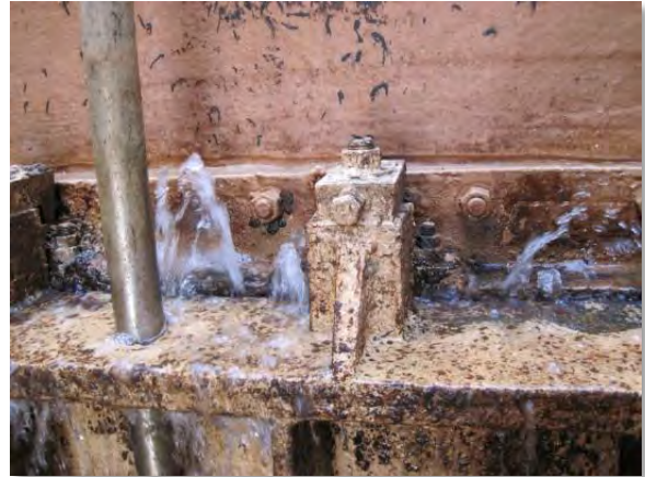
Photo 3-87. Close-up of leak on sluice gate at northeast corner of CCC.
