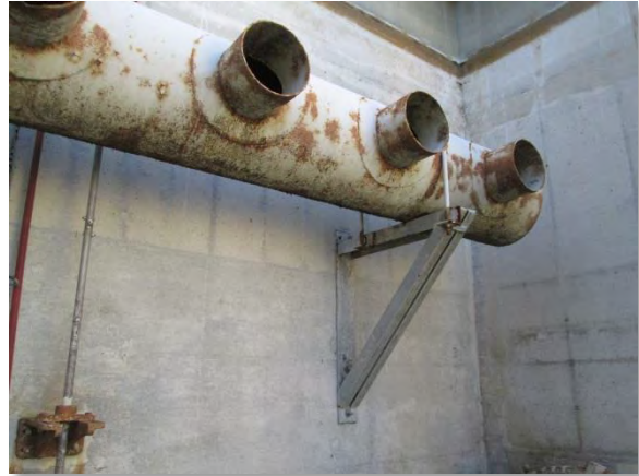
Photo A-18. Steel manifold pipe with minor coating failure and corrosion.
