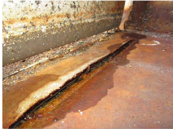
Photo 3-37. Deteriorated sealant at expansion joint near west end of SST 2 with evidence of possible infiltration.
