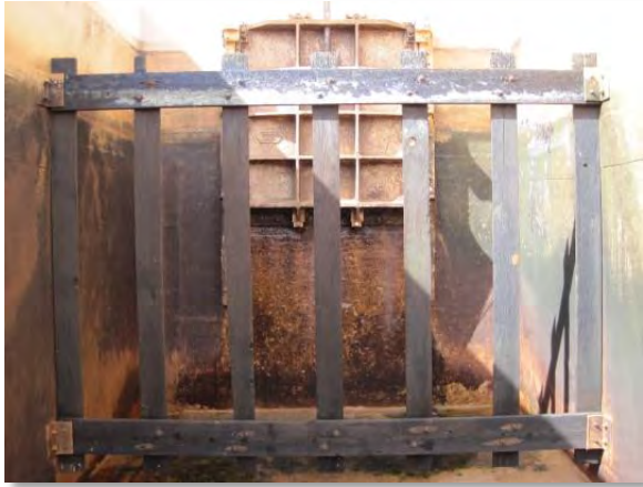
Photo 3-70. The bolts and supports of the baffles were in VANDA Level 1 condition.
