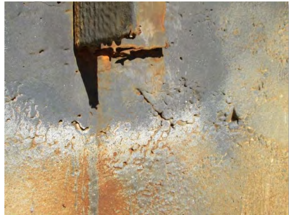
Photo A-26. Rock pockets in PC 1 wall at approximate 10:30 position.
