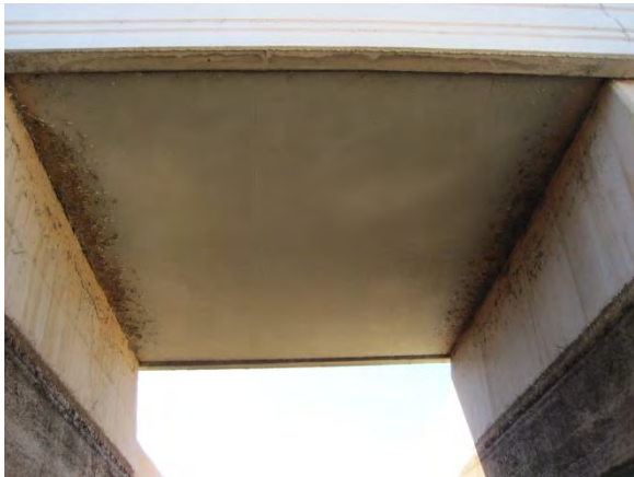
Photo 3-74. No cracks or spalls were observed on the underside of the pedestrian bridge.
