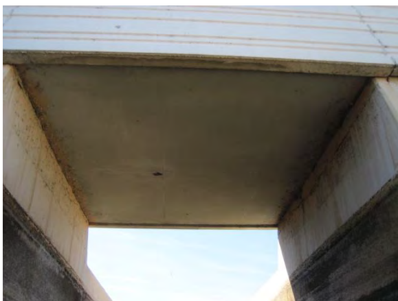
Photo 3-76. No cracks or spalls were observed on the underside of the pedestrian bridge.
