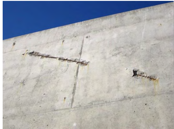
Photo 3-21. Detail view of spall near top of midpoint of west wall.
