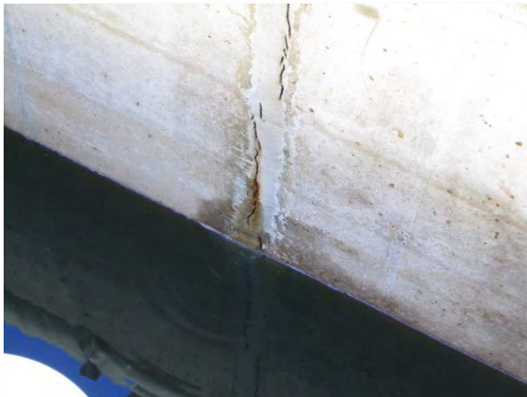
Photo 3-50. Typical sealant in expansion joint with shrinkage and gaps.
