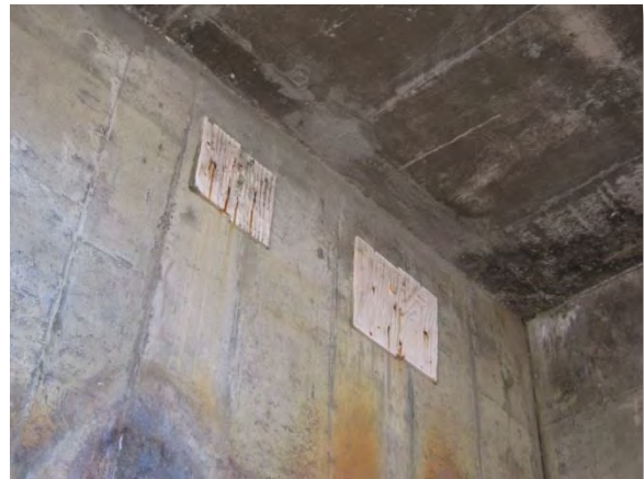
Photo A-63. Wood embedded in wall at northeast corner.
