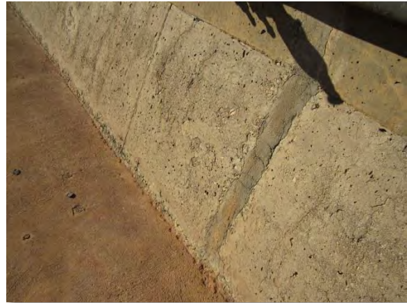
Photo A-53. Construction joints on west wall with deteriorating mortar overlay (typical).
