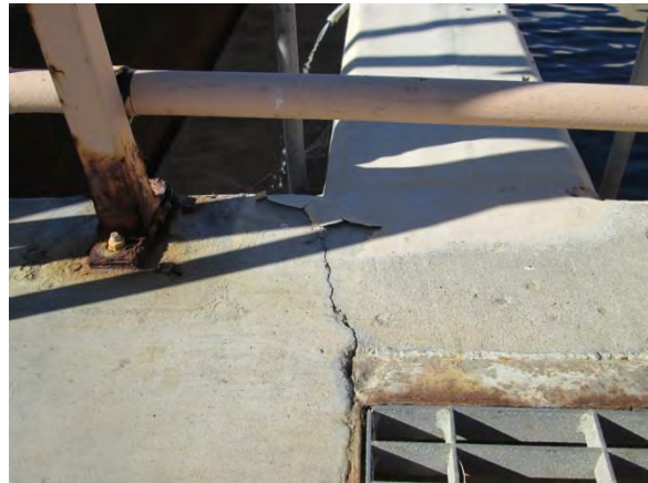
Photo 3-75. Crack observed on the deck level at the northeast corner of the north pass.
