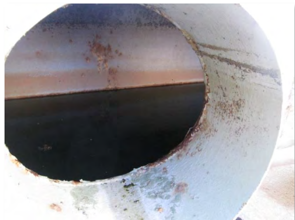
Photo A-16. Steel manifold pipe with minor coating failure and corrosion.
