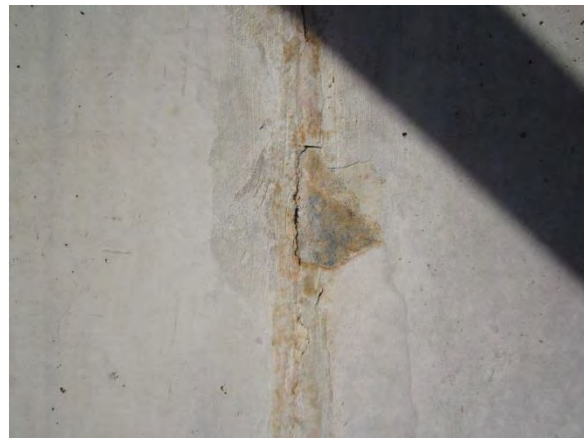
Photo A-40. Detail of possible seepage through construction joint near midpoint of north wall.
