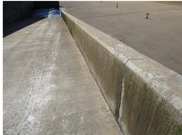
Photo 3-17. Cracks in a few locations are visible on both sides of the wall and appear to extend through it.
