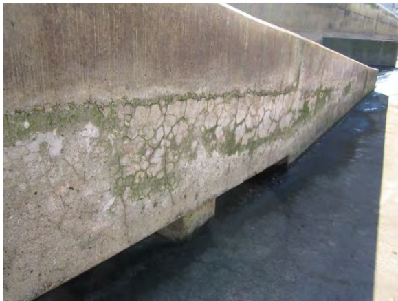
Photo 3-15. Cracked surface layer near bottom of ramp.
