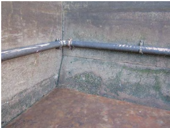
Photo A-58. Southwest corner of West FEB with isolated rock pockets.
