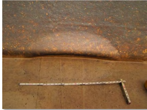
Photo 3-71. Approx. 24-inch-long by 12-inch-wide blister on north wall of north pass.
