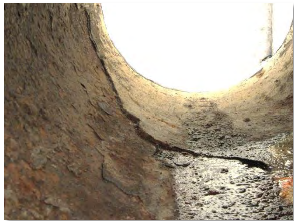
Photo A-47. Damage to cement mortar lining inside inlet tee at east wall.
