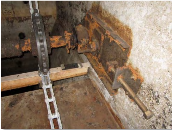
Photo A-44. Coating failure and minor corrosion on brackets for skimmer system.
