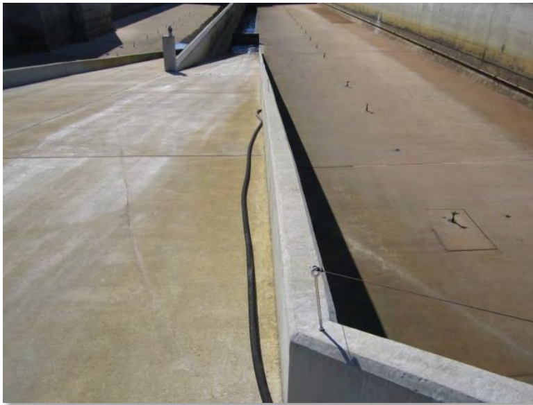
Photo 3-28. North end of wall along ramp. Low height of wall presents a fall hazard.
