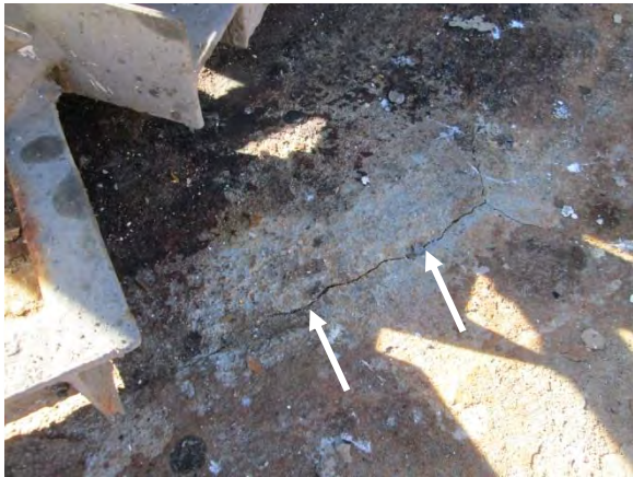
Photo A-25. Cracks near center column have separated about 1/8 of an inch.
