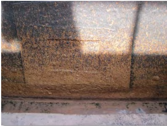
Photo 3-82. Approx. 24-inch-long by 24-inch-wide coating repair section. This section is hollow, which suggests the coating is not properly adhered.
