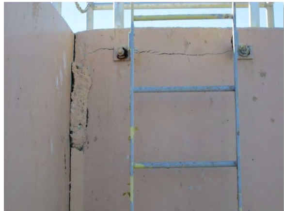
Photo C-16. Broken concrete at top of effluent tower.
