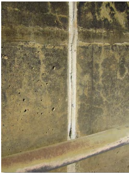
Photo A-54. Typical condition of expansion joint sealant on walls.
