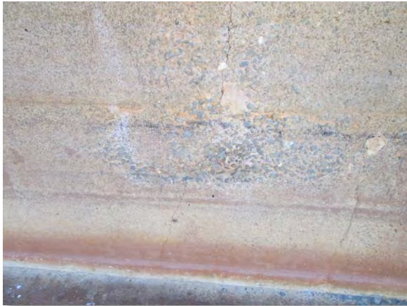
Photo 3-58. Typical exposed aggregate and cracking on lower wall.
