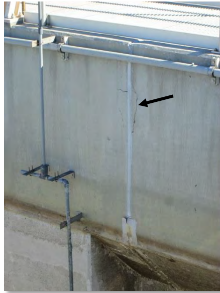
Photo C-8. Spalling concrete adjacent to expansion joint.
