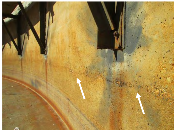
Photo 3-63. Rock pockets in PC 1 wall at approximate 10:30 position.
