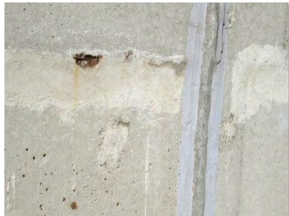
Photo 3-45. Spalling mortar with moderate corrosion of reinforcing steel near expansion joint 396 feet south of north wall.
