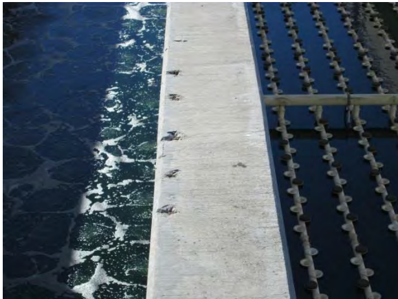
Photo 3-46. Exposed ends of reinforcing bars at top of wall between ASTs 1B and 1C.
