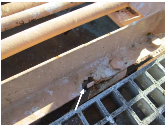
Photo 3-68. Holes through lower members of catwalk truss. Corrosion damage has been painted over.
