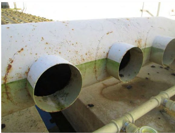
Photo 3-54. Steel manifold pipe with minor coating failure and corrosion.
