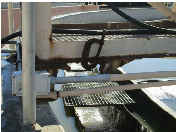
Photo C-17. Apparent broken welds on catwalk.
