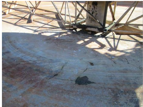
Photo 3-61. Minor apparent groundwater infiltration from cracks in floor.
