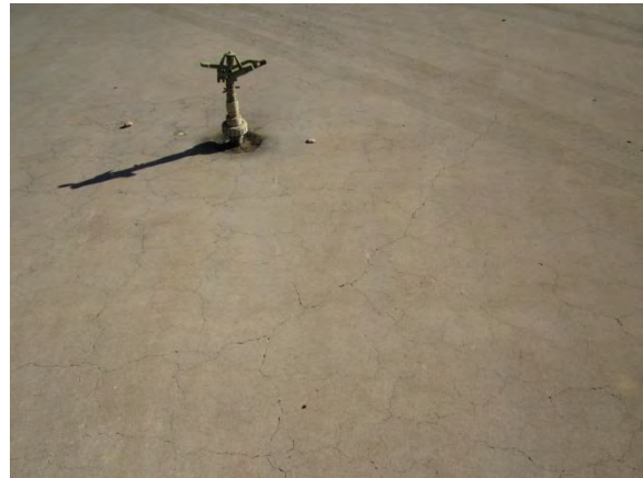
Photo 3-4. Typical cracking on West FEB floor.
