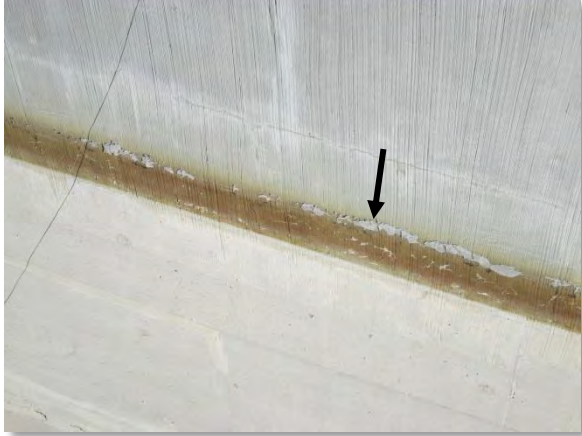
Photo C-3. Deteriorating mortar overlay at top of west wall.
