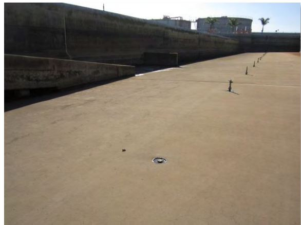
Photo A-67. Missing sprinkler head in West FEB.
