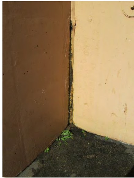
Photo C-12. Effluent tower separating from clarifier wall.
