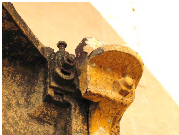
Photo 3-88. Minor damage to the coating on the gate guide.
