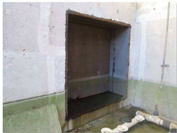
Photo 3-55. Minor coating failure and corrosion on sluice gates and frames.
