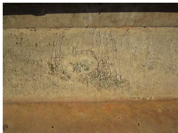
Photo 3-12. Typical concrete surfaces along toe of west wall with intermittent areas of exposed aggregate.
