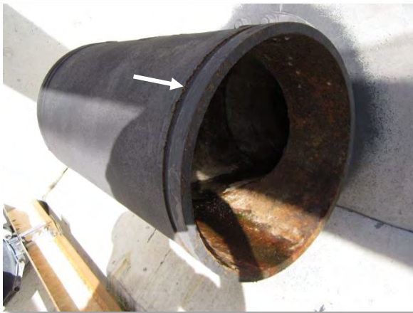
Photo A-46. Inlet tee at east wall. Arrow denotes minor coating failure and surface corrosion.
