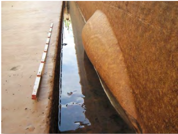
Photo 3-72. Approx. 48-inch-long by 12-inch-wide blister on south wall of north pass.
