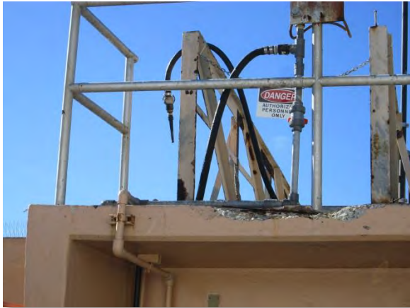
Photo C-13. Spalling on edge of landing at top of stairs.
