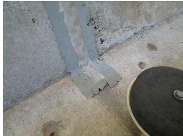
Photo 3-51. Overlay sealant on expansion joint with gaps at ends (typical).
