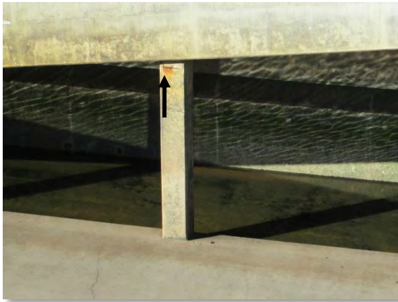
Photo C-19. Spalling on column.
