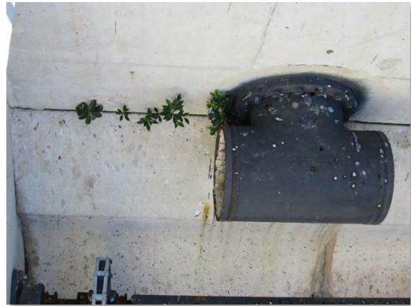
Photo C-31. Plants growing from gap behind fill concrete at east wall.
