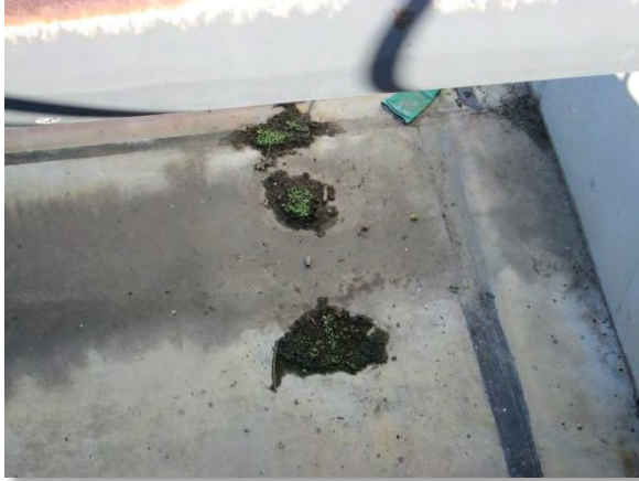
Photo C-34. Weeds growing from expansion joints.
