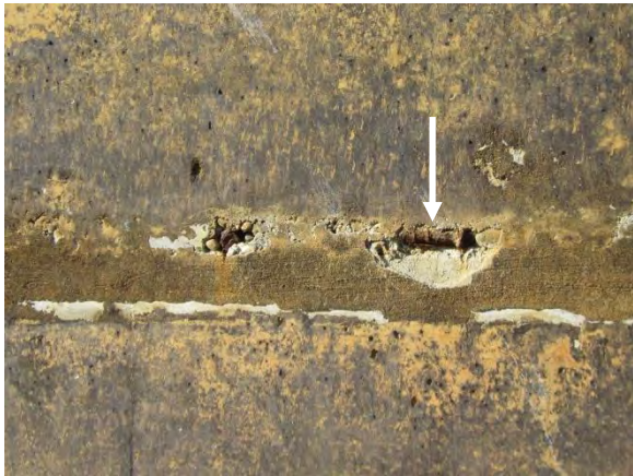
Photo 3-5. Broken mortar and exposed reinforcing bar at some locations along construction joint in west wall.
