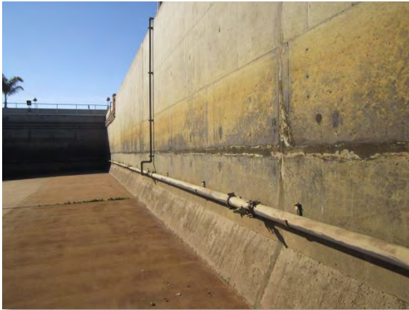
Photo A-52. Construction joints on west wall with deteriorating mortar overlay (typical).
