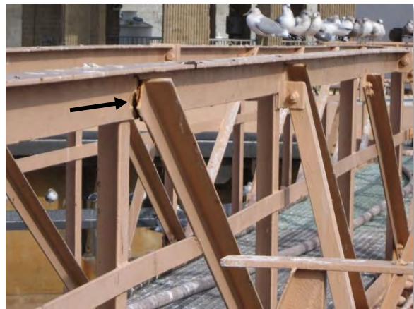
Photo A-32. Loose bracing on PC 1 catwalk truss due to broken or corroded welds.
