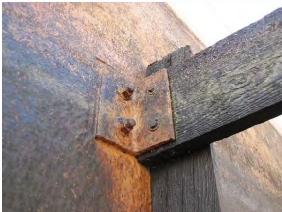
Photo 3-80. The coating on the brackets for the wooden baffles is in good condition.
