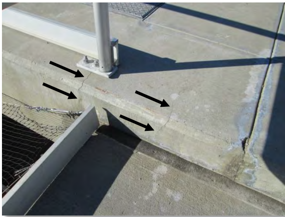
Photo A-37. Cracking of platform above west end of SST 2.
