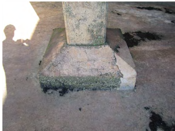
Photo 3-27. Cracked concrete at base of column with apparent repair at right.
