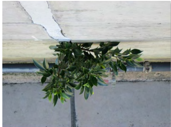
Photo C-24. Weeds growing from sealant in east wall.
