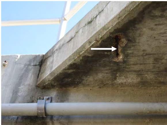
Photo C-36. Spalling on underside of platform at southeast corner.
