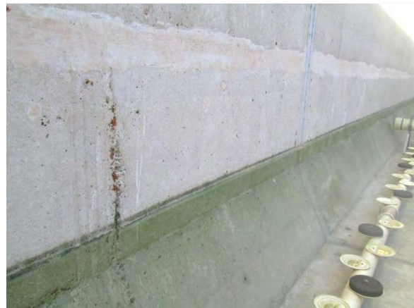
Photo 3-49. Exposed steel (possible vertical reinforcing bar) about 4 feet above floor on west wall and about 95 feet south of north wall.
