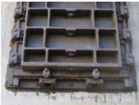
Photo A-15. Minor coating failure and corrosion on sluice gates and frames.
