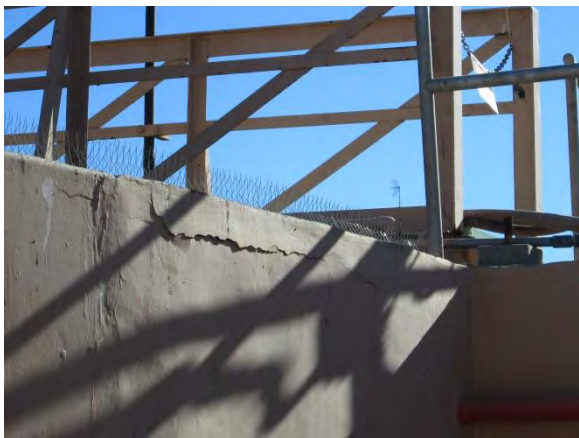
Photo 3-64. Broken concrete at top of PC 1 wall near stairway.
