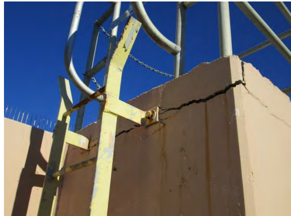
Photo C-10. Broken concrete at top of effluent tower.
