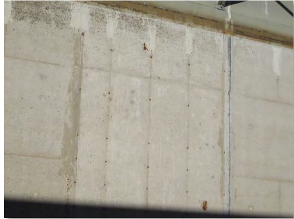
Photo A-10. Multiple small sources of corrosion staining on west wall.
