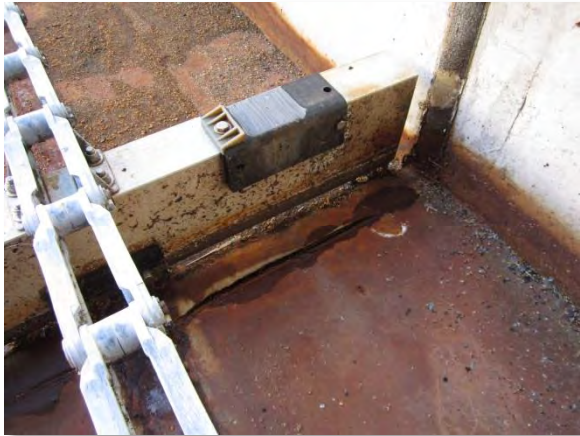
Photo 3-36. Deteriorated sealant at expansion joint near west end of SST 2 with evidence of possible infiltration.
