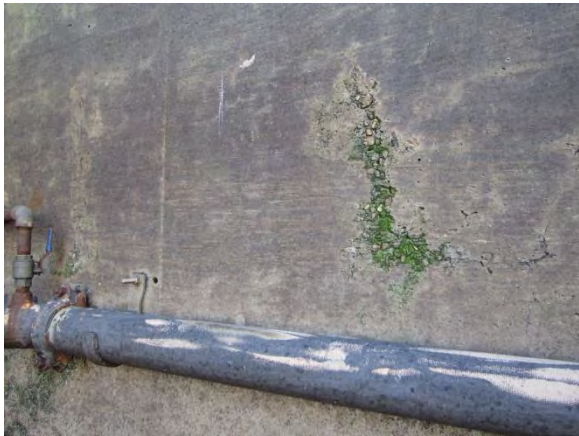
Photo 3-13. Typical isolated rock pocket in west wall near southwest corner.
