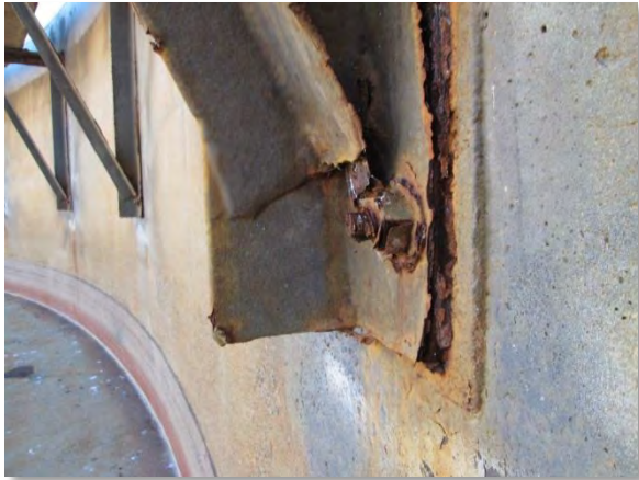
Photo A-29. Typical coating failure and corrosion on PC 1 launder brackets.
