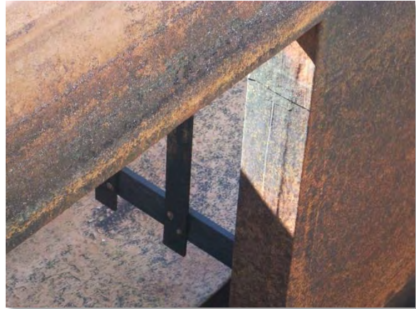
Photo A-73. Coating condition at east end of CCC.
