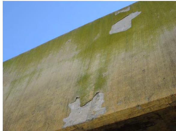
Photo 3-14. Overlay layer spalling off of edge of wall and ramp.
