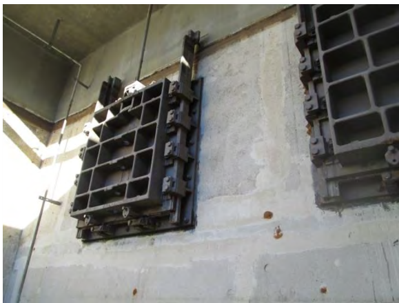
Photo A-11. Multiple small sources of corrosion staining on north wall.
