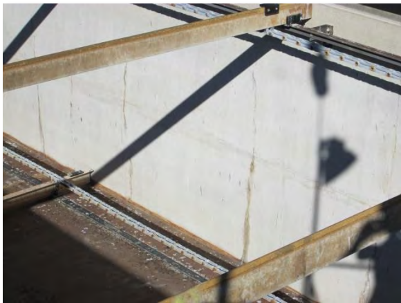
Photo C-28. Vertical cracks every few feet along length of north wall (similar to SST 2).
