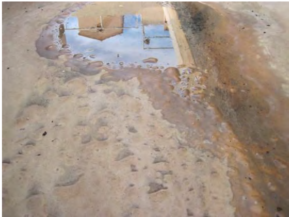
Photo 3-78. Blisters on floor were observed along a 40-foot-long section of the floor.
