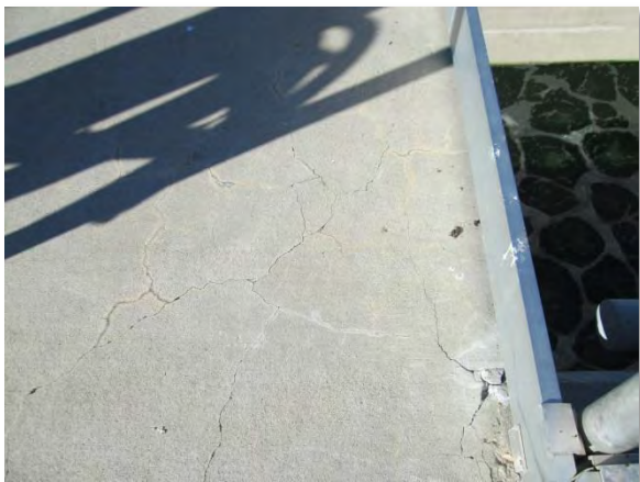
Photo C-5. Cracking on top surface of walkway.
