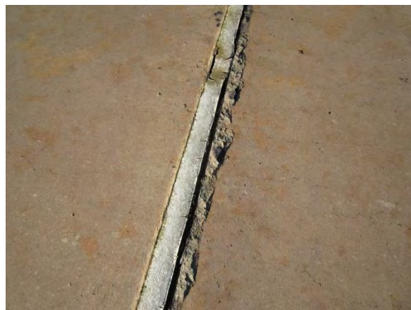
Photo 3-8. Spalled concrete adjacent to expansion joint in floor.
