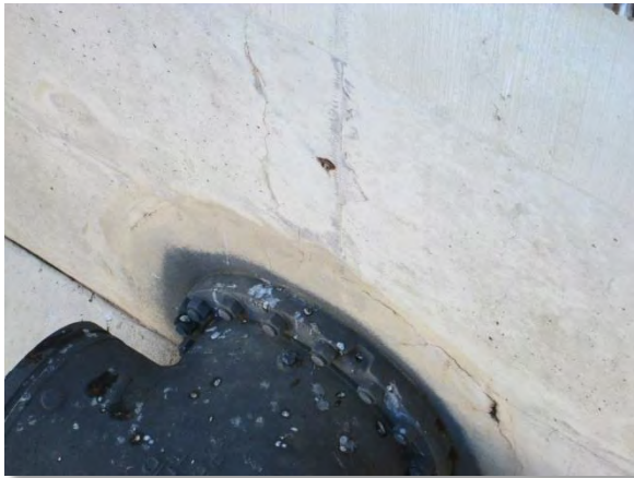
Photo C-27. Cracking in east wall above inlet tee.
