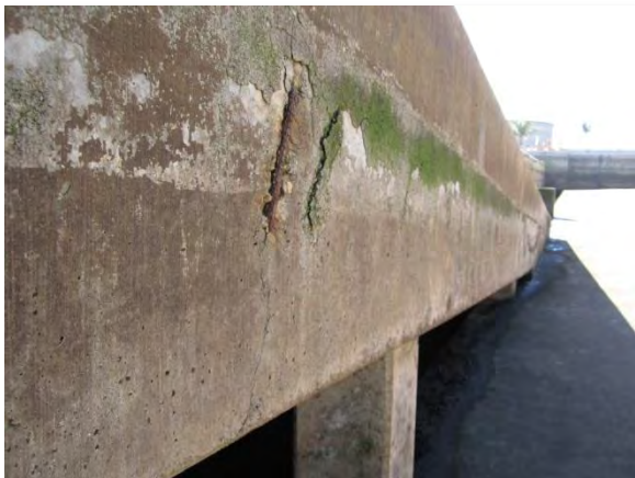
Photo 3-18. Typical minor spalling on outside of ramp.
