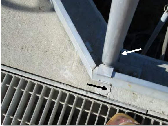
Photo C-7. Cracking at southeast corner of basin.
