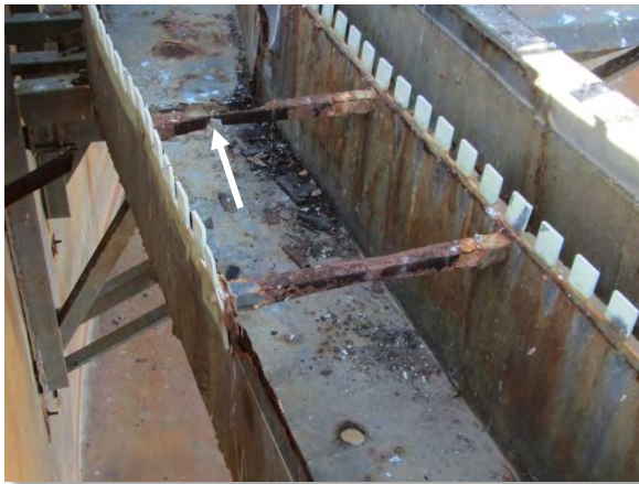
Photo 3-66. Severe corrosion of cross-braces across top of PC 1 launders.
