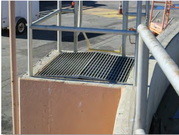
Photo C-11. Grating on top of effluent tower not seated properly, reportedly due to corrosion products.
