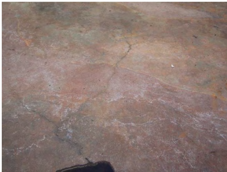
Photo 3-35. Typical minor cracking on floor of SST 2. Possible infiltration visible at bottom of image.
