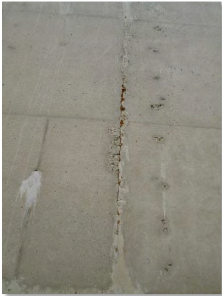
Photo A-9. Loss of mortar over construction joint on east wall about 350 feet south of north wall.
