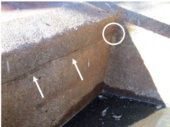
Photo 3-62. Grout or mortar joint at the center sludge pit. A short section of apparently exposed reinforcing steel was also visible (circle).
