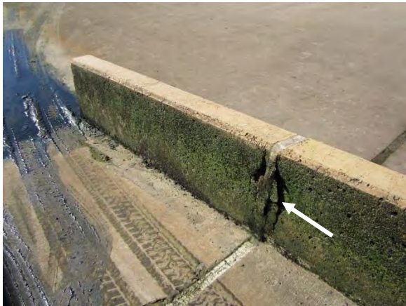
Photo 3-9. Spalled concrete adjacent to expansion joint in wall at bottom of ramp.
