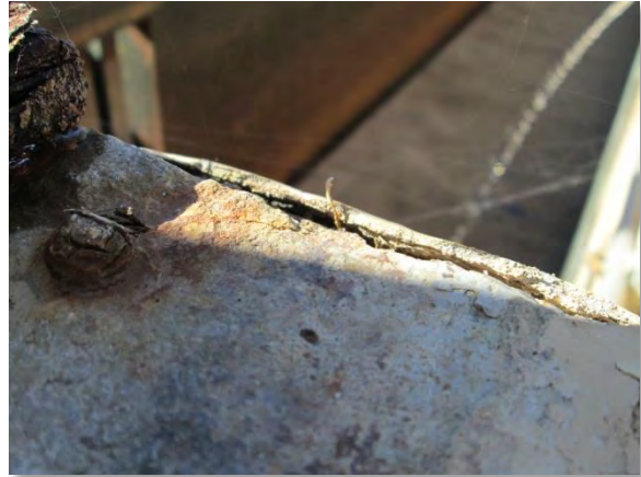
Photo A-80. Coating delamination at northeast corner.
