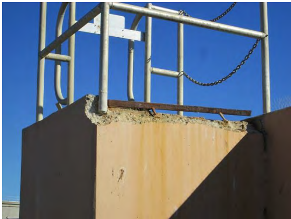
Photo C-15. Broken and missing concrete at top of effluent tower.
