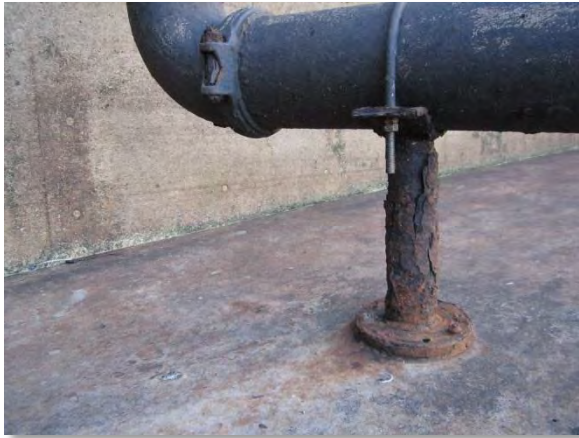
Photo A-64. Corroding pipe support near south wall.
