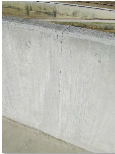
Photo C-20. Typical crack in east wall (appears to pass through wall).
