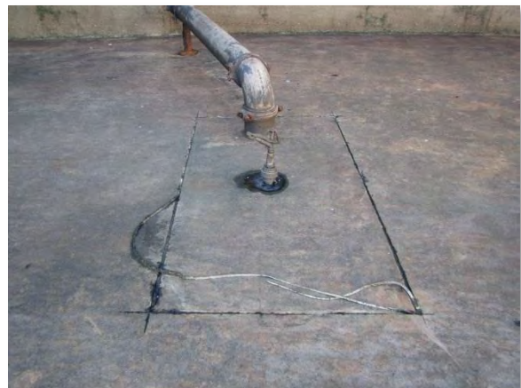
Photo 3-23. Joints around sprinkler near south end of FEB, with sealant coming loose.
