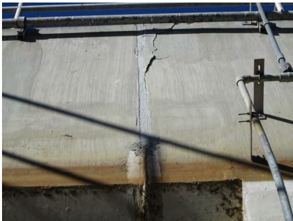
Photo 3-52. Spalling concrete adjacent to expansion joint on west wall about 303 feet south of north wall.
