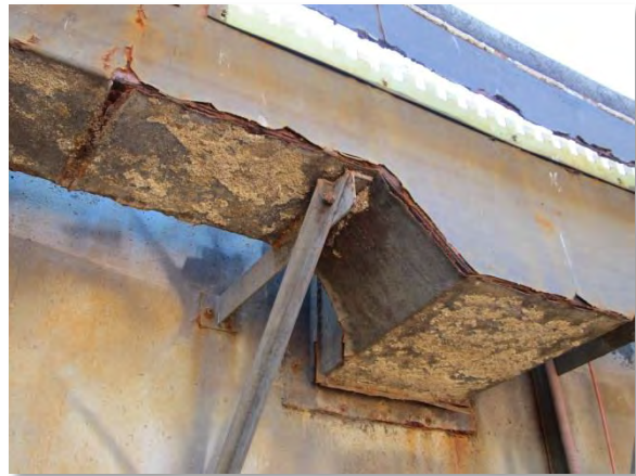
Photo 3-67. Typical coating failure and corrosion at edges on PC 1 launders.
