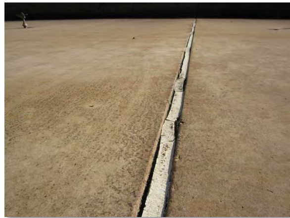
Photo A-55. Typical condition of expansion joint sealant on floor.
