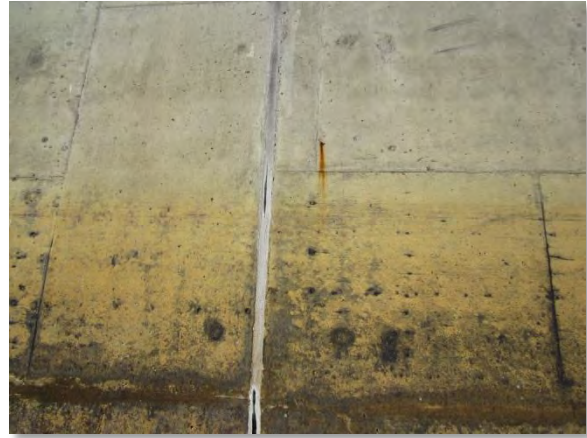
Photo A-61. Typical minor corrosion staining on west wall.
