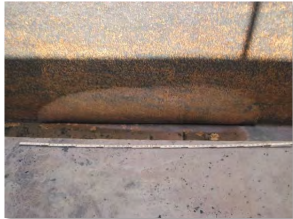
Photo 3-83. Approx. 54-inch-long by 12-inch-wide coating blister on north wall of south pass.
