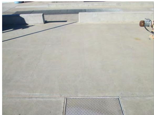
Photo C-26. Cracking in slab over west end of basin (more extensive than SST 2).
