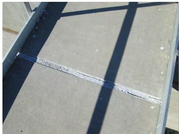
Photo C-6. Gaps in sealant in expansion joint in walkway.
