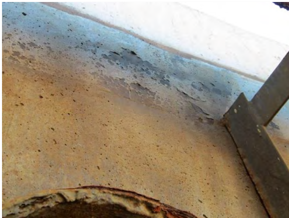
Photo A-27. Deteriorated coating on upper interior surfaces of wall.
