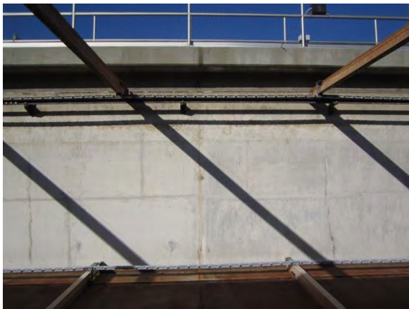
Photo A-39. Evidence of possible seepage through construction joint near midpoint of north wall (south wall similar).
