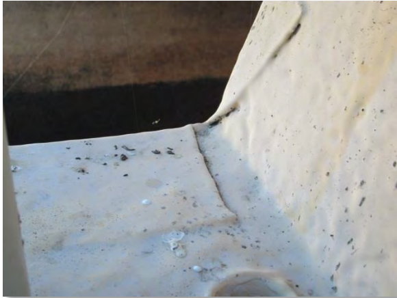
Photo A-79. Coating termination at top of south wall near walkway.
