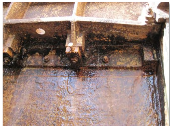
Photo 3-89. Minor leaking of the inlet sluice gate.
