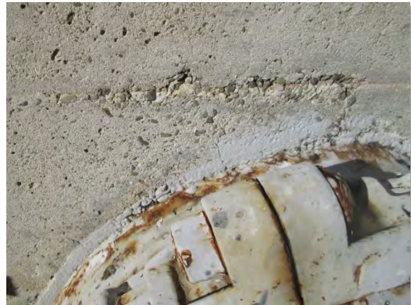
Photo A-14. Rock pocket above manifold pipe penetration about 305 feet south of north wall.
