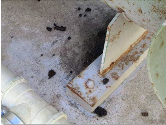
Photo A-17. Steel manifold pipe with minor coating failure and corrosion.
