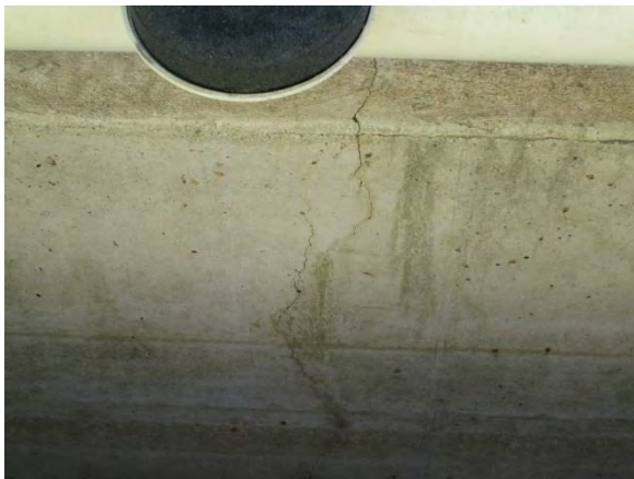
Photo 3-44. Typical cracking on floor and walls of center trough.
