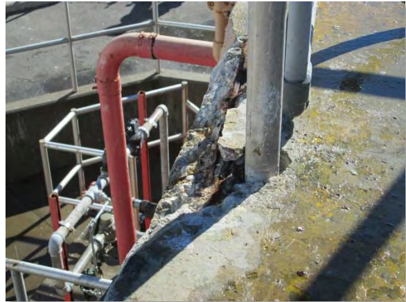
Photo C-14. Spalling on edge of landing at top of stairs.
