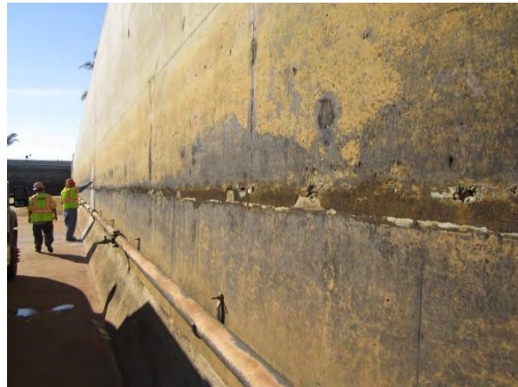
Photo 3-6. Reinforcing bar exposed at construction joint intermittently over approximate 50-foot length.
