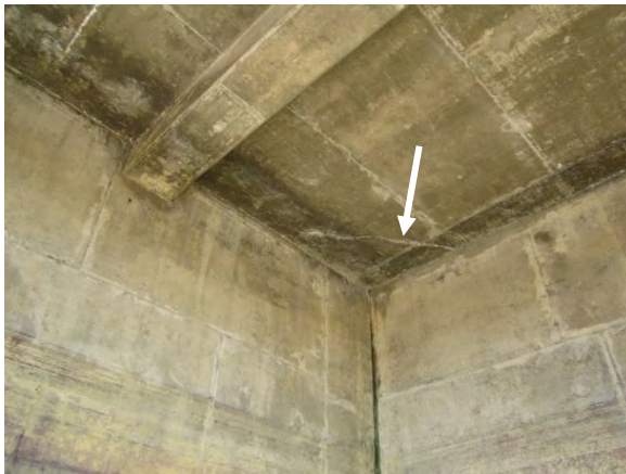
Photo A-62. Minor cracking and efflorescence on bottom of platform at northwest corner of West FEB.
