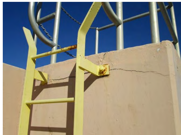
Photo 3-65. Broken concrete at top of effluent tower (typical).
