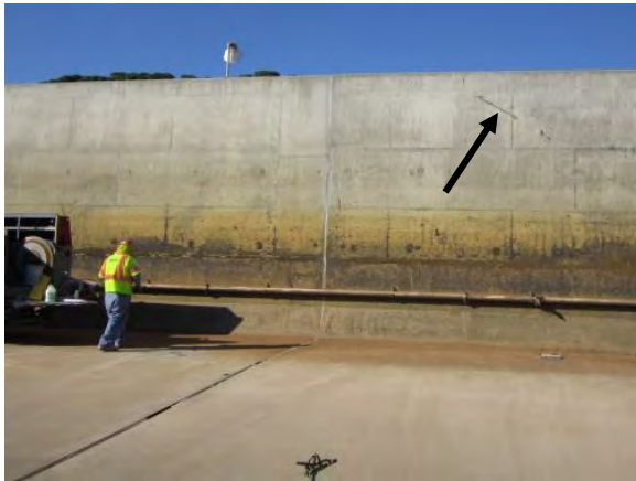
Photo 3-20. Location of spall near top of midpoint of west wall.
