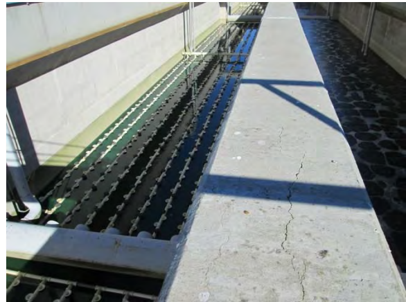
Photo 3-47. Cracking on top surface of wall between ASTs 1B and 1C (typical).
