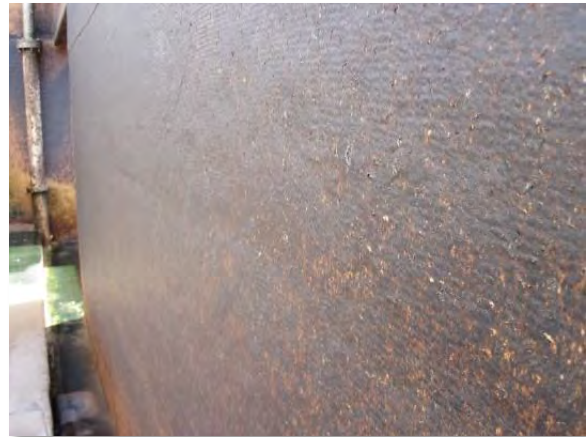
Photo 3-73. Area of hollow coating on south wall of north pass suggests the coating is not properly adhered.
