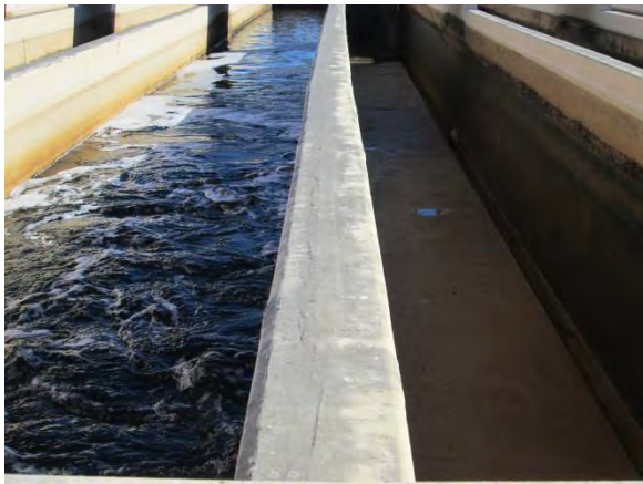
Photo A-74. Coating condition at top of north wall of north pass (North CCC at left).
