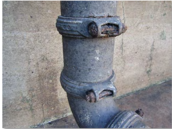
Photo A-65. Corroded hardware on Victaulic couplings for pipe at south wall.
