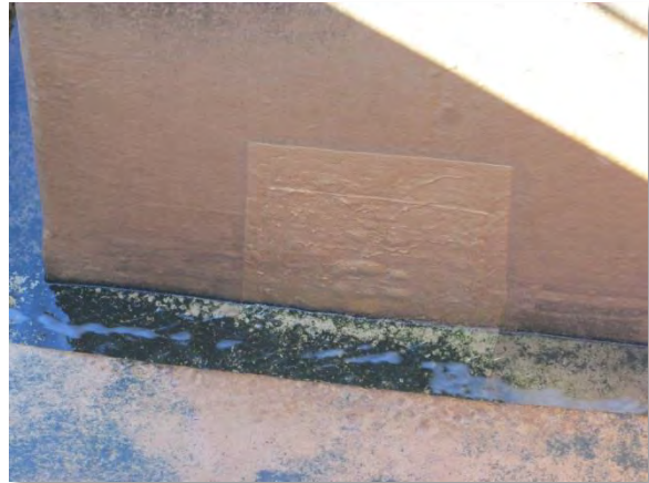
Photo A-76. Typical coating patch.
