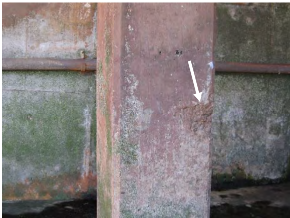
Photo 3-26. Damaged corner on column.
