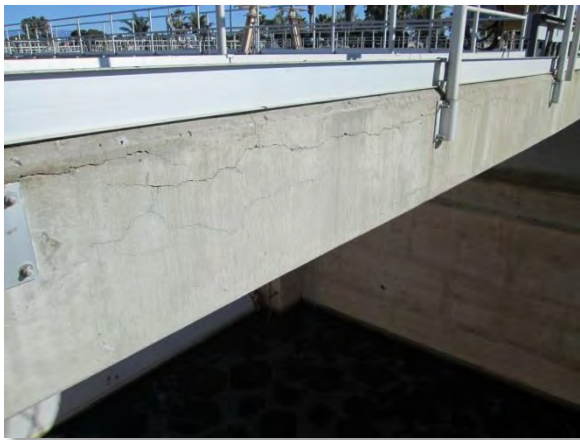
Photo C-1. Cracking on edge of walkway.
