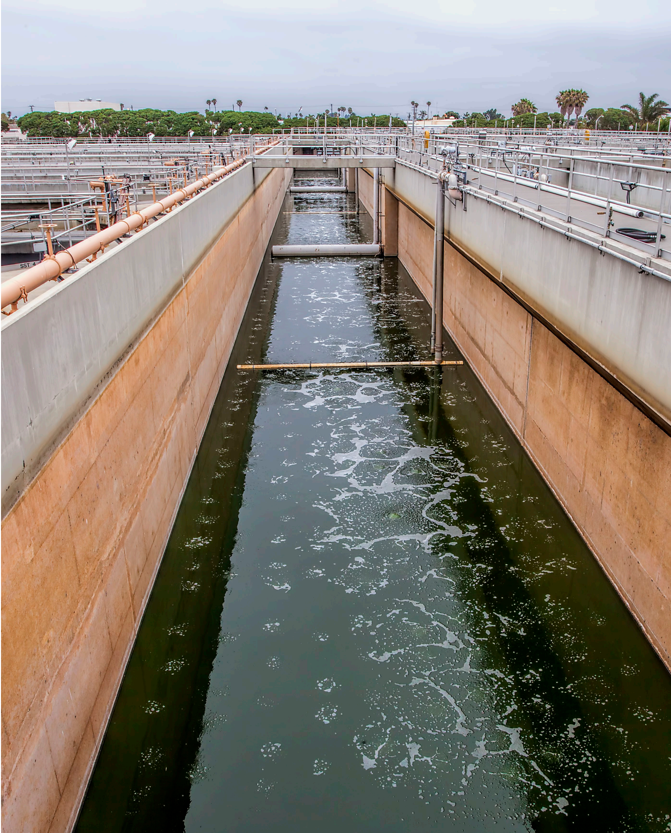
Activated sludge tanks
