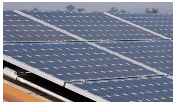
Solar panel array
