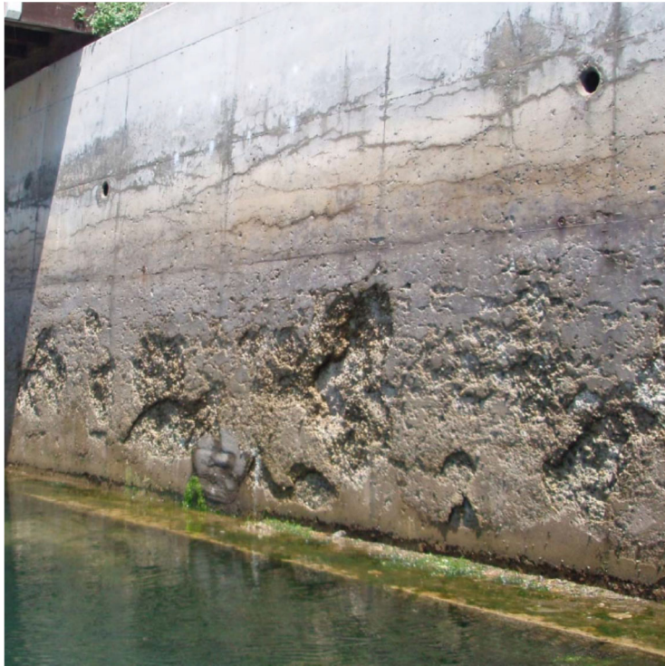
Figure 5 - Spalling and surface erosion on Zurn wall [from TranSystems (2017)]
