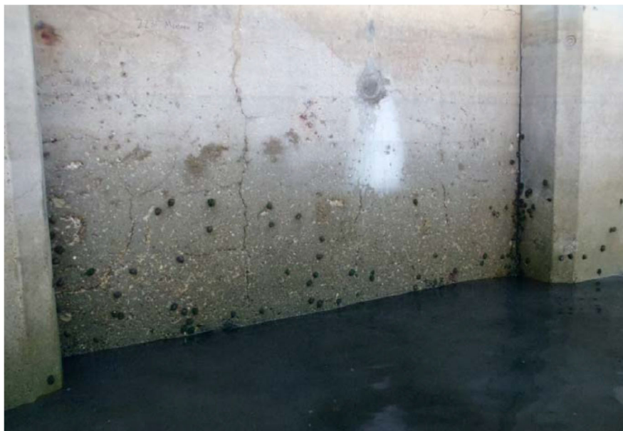
Figure 6 - Surface erosion and vertical cracking on a Boise wall panel [from TranSystems (2011)]
