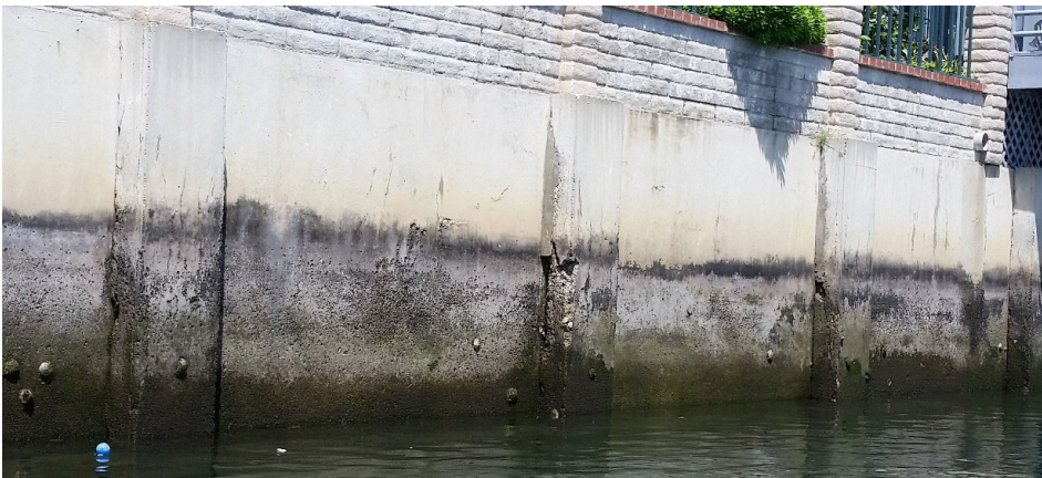
Figure 4 - Surface erosion/marine attack on Boise wall panels with cracking and spalling at pilasters
