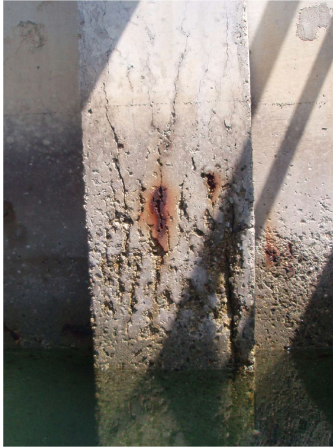
Figure 7 - Vertical cracking and spalling on Boise wall pilaster [from TranSystems (2017)]
